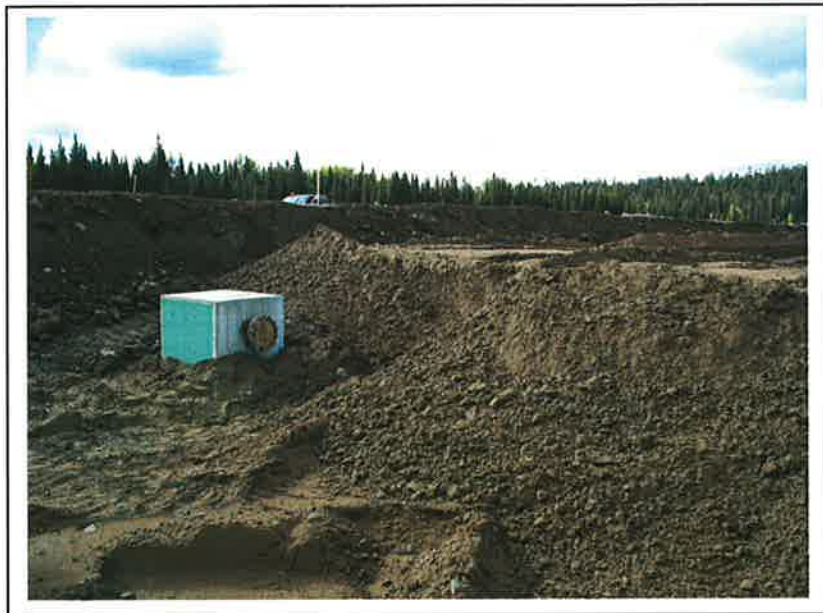
PHOTO 10 – Upstream toe drain outlet at the South Embankment. To be completed in 2009.
