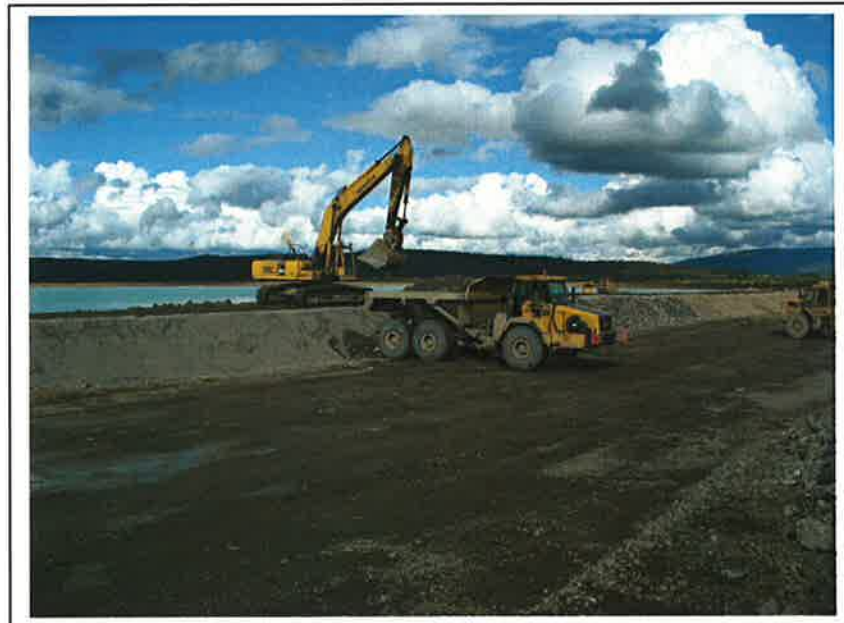
PHOTO 2 – Downstream components of TSF, Zone C (foreground), Truck is placing Zone T on top of Zone F, Excavator is sitting on Zone S at 954m
