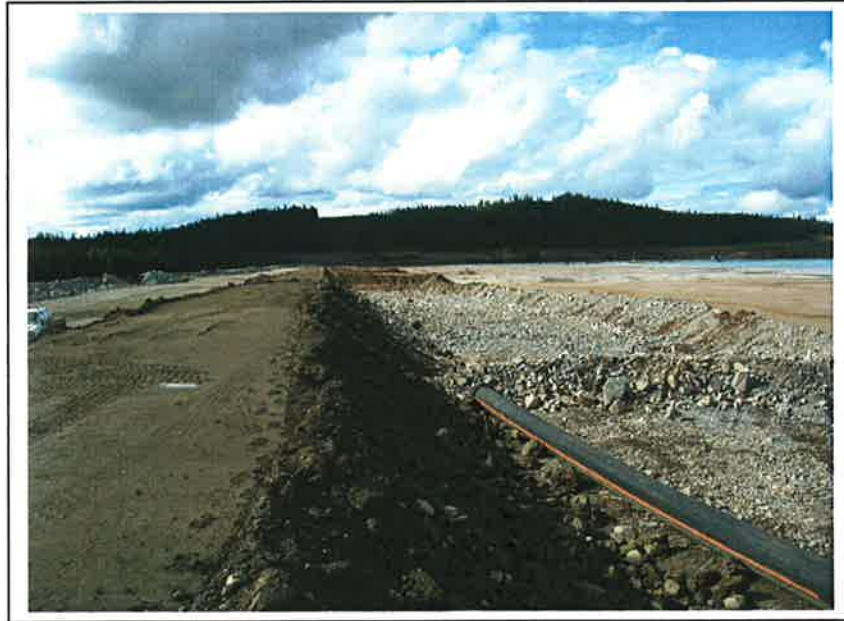
PHOTO 1 – Components of the TSF, Zone S (left) Zone U (centre) and Tailings Beach (right)
