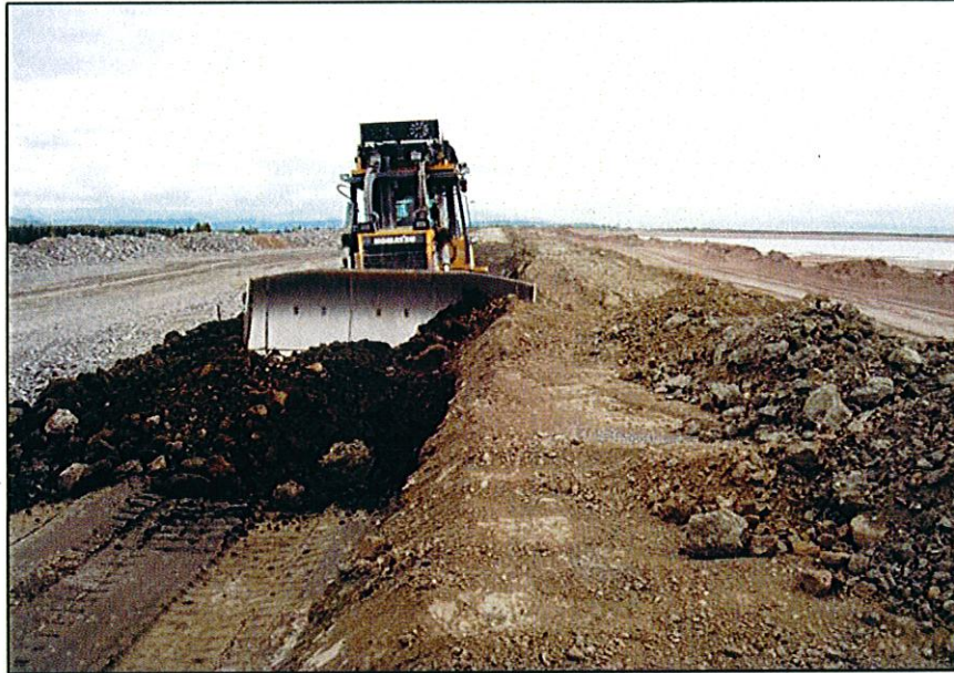
PHOTO 43 – Keying in to the till in the underbuilt sections, to sufficiently blend the new and existing tills.
