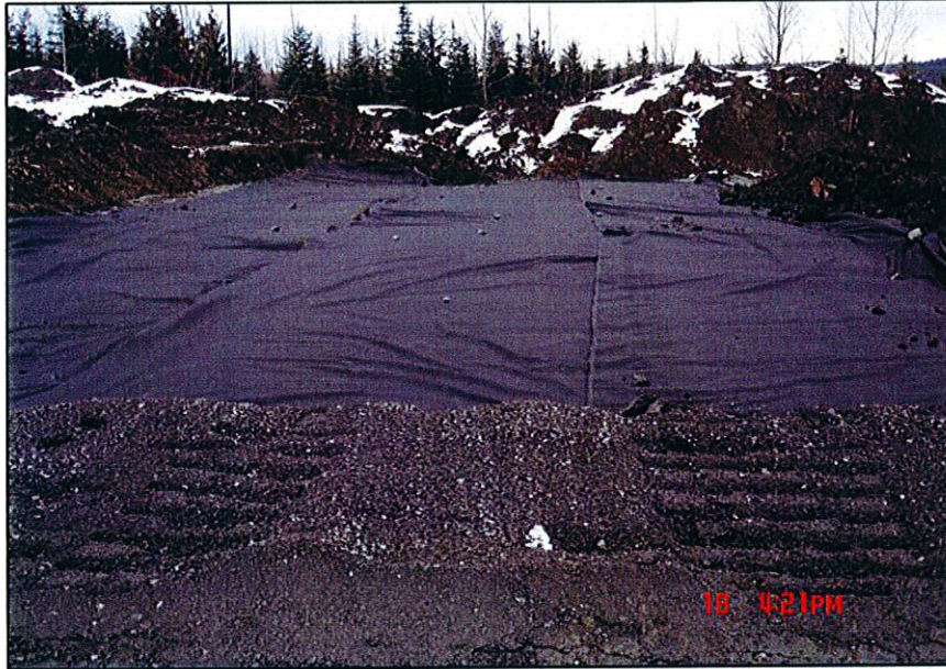
PHOTO 15 – Placement of geotextile cloth ovetop of the original ground (competent till) prior to placement of Zone F material along the Perimeter Embankment
