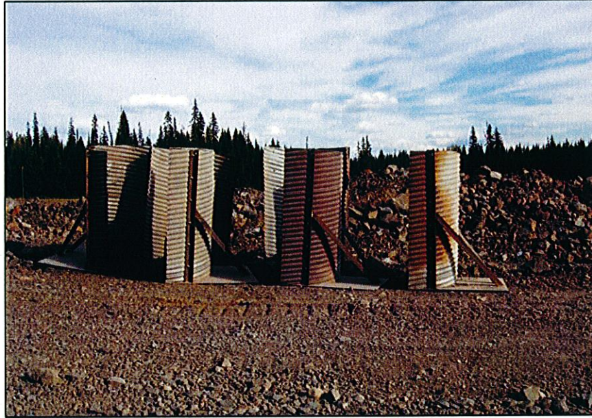
PHOTO 11 – Protective covers for the piezometers located at the Main Embankment toe, to shield them from loose Zone C material
