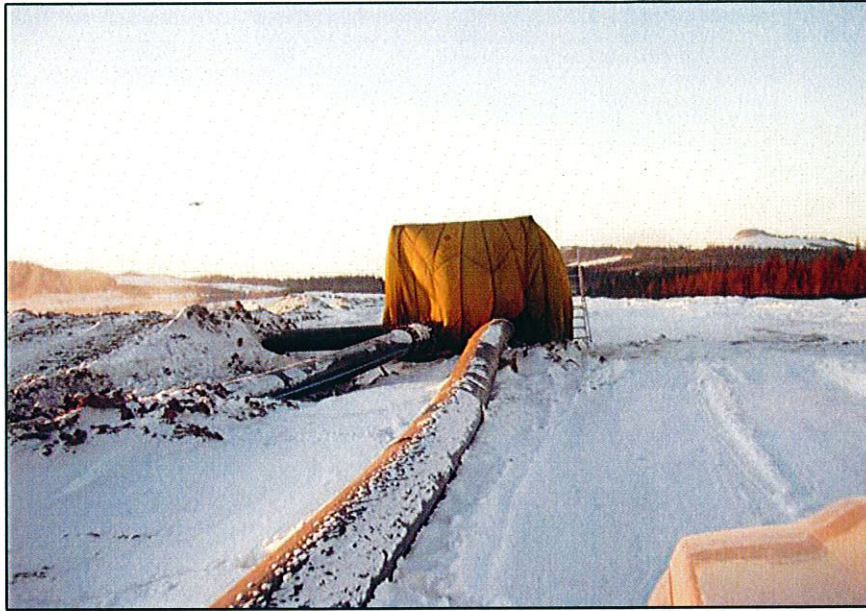
PHOTO 31 – Heating the tailings pipeline valves during the winter months to prevent them from freezing
