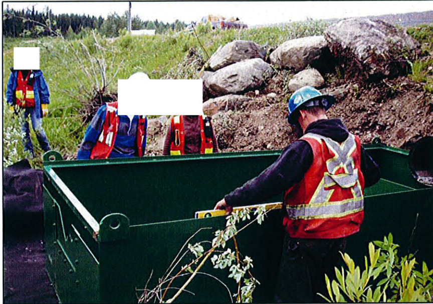
PHOTO 35 – Leveling the weir box, which will be used to measure flows exiting the Main Seepage Pond once a permit is received.
