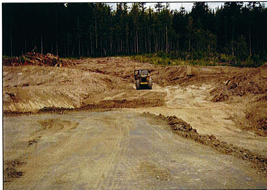
PHOTO 46 – Preparing the north end of the South Embankment for placement of Zone S material.
