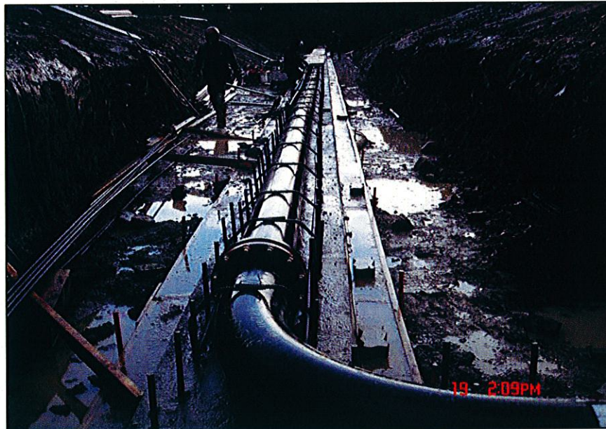
PHOTO 16 – Steel pipe to be joined to the Perimeter Embankment upstream toe drain
