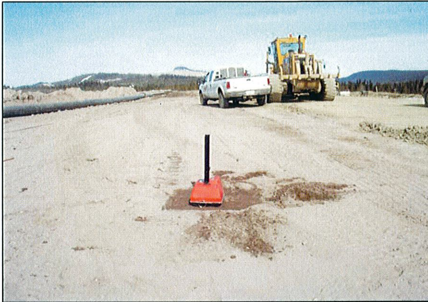
PHOTO 53- Performing a compaction test on the Main Embankment U zone with the nuclear densometer.
