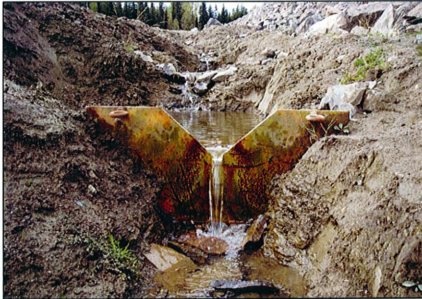
PHOTO 33 – V- notch weir used to measure flows at the corner downstream of the Main and South Embankments.
