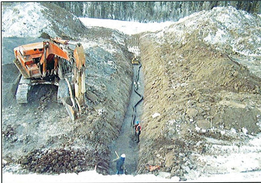
PHOTO 25 – Installing the longitudinal drain to be connected to the South Embankment toe drain
