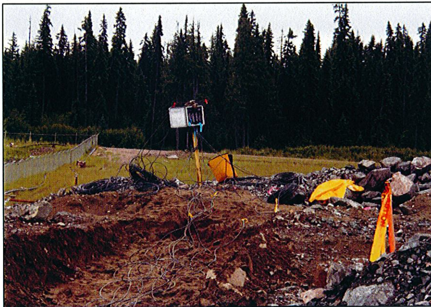
PHOTO 12 – Placing the piezometers in a read-out box for more efficient data collection
