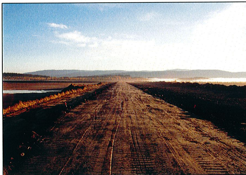
PHOTO 48 – Looking eastward along the Main Embankment with Zone S up to 951 m.
