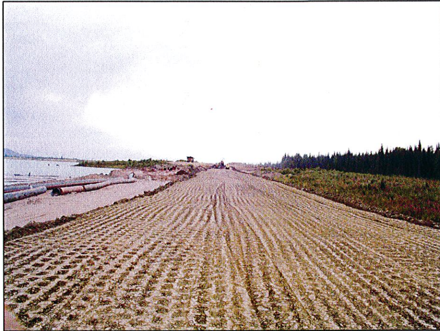
PHOTO 21 – Scarifying the Zone S material at the South Embankment with a sheepsfoot prior to placing the next lift.
