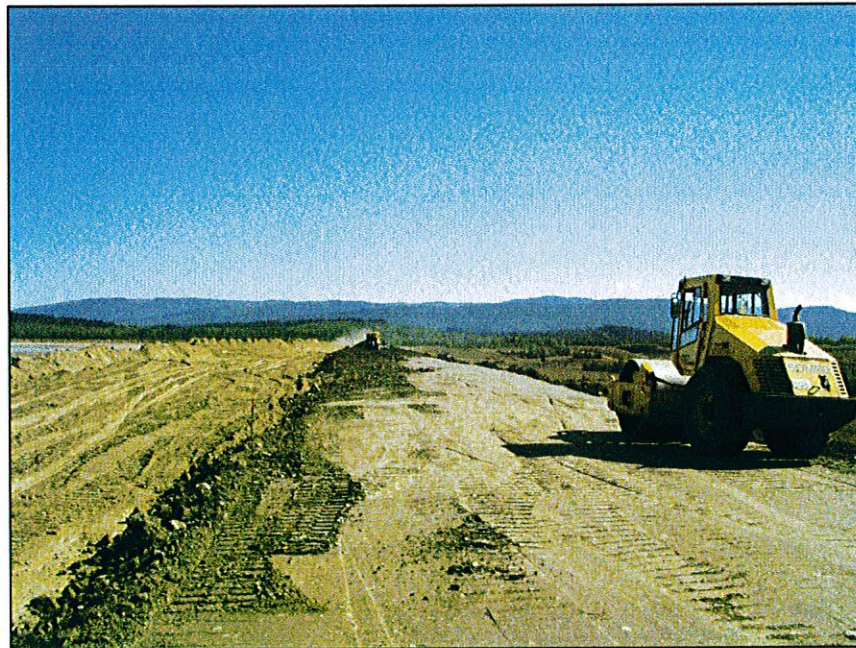
PHOTO 24 – The vibratory smooth drum compacting Zone S material on the Main Embankment.
