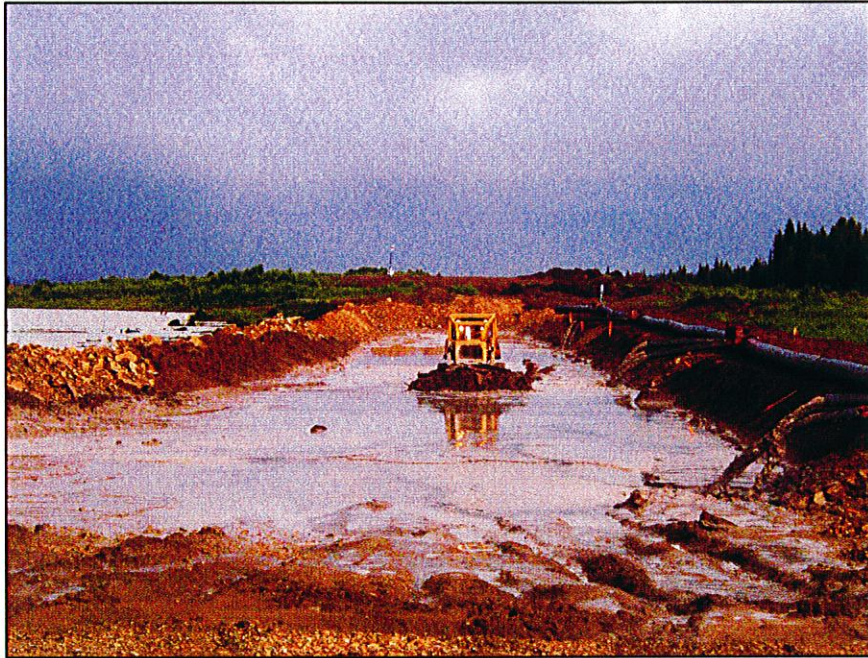
PHOTO 11 – Using a dozer in the sand cell at the South Embankment to distribute and compact the tailings sand.
