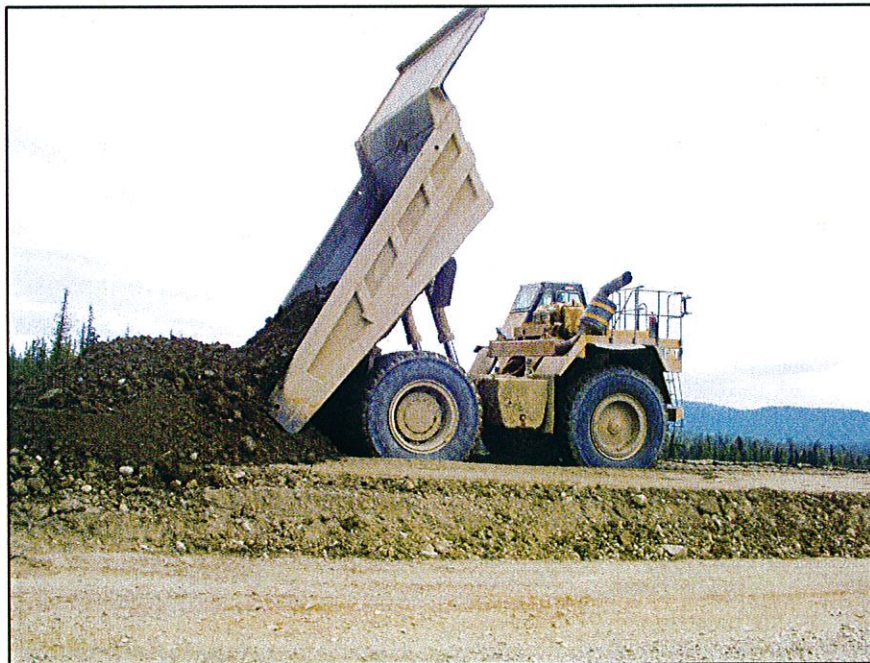
PHOTO 28 – Placing Zone S material with a 777 haul truck on the Perimeter Embankment.
