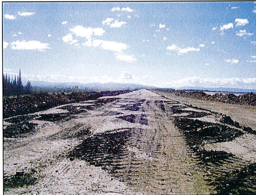
PHOTO 20 – Scarifying the Zone S material at the Perimeter Embankment with a dozer prior to placing the next lift.
