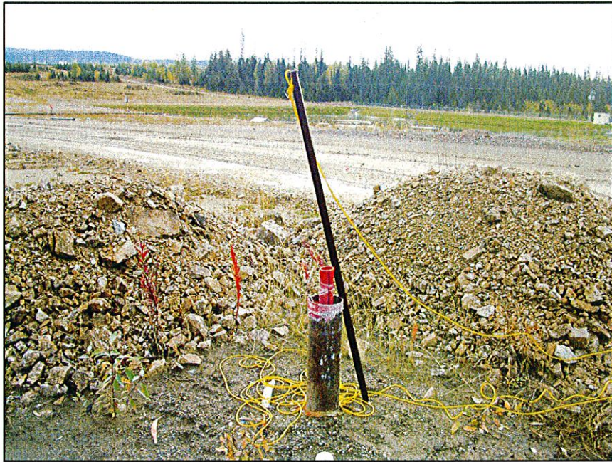
PHOTO 33 – A “poorboy” was used to ensure that there were no “pinch points” in the inclinometers.
