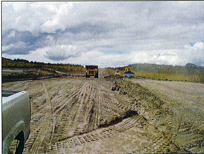
PHOTO 19 – Placing sand from the Cyclone sand stock pile on the Perimeter Embankment as Zone U.
