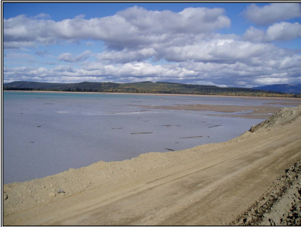
Photo 17: Lack of Established Beach – Perimeter Embankment in Background
