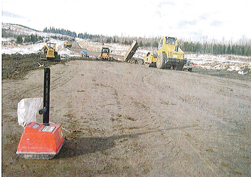
PHOTO 13 – Construction of Zone S material at the perimeter embankment and quality control test by nuclear gauge instrument.
