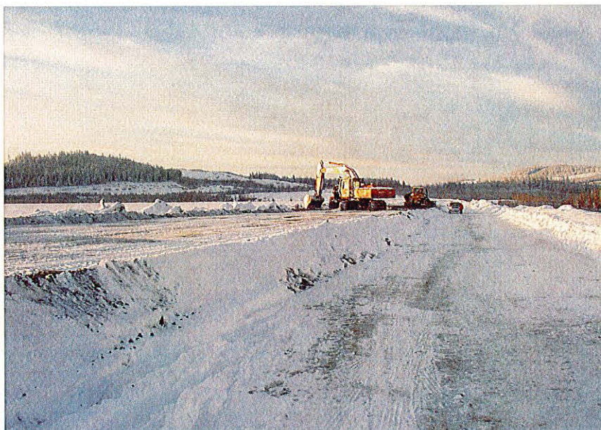
PHOTO 16 – Scraping the fill surface during winter with a excavator as part of the foundation preparation procedure.
