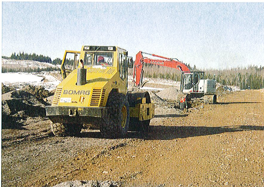
PHOTO 11 – Compaction of Zone F material with a 10 tonnes smooth drum vibrating compactor.
