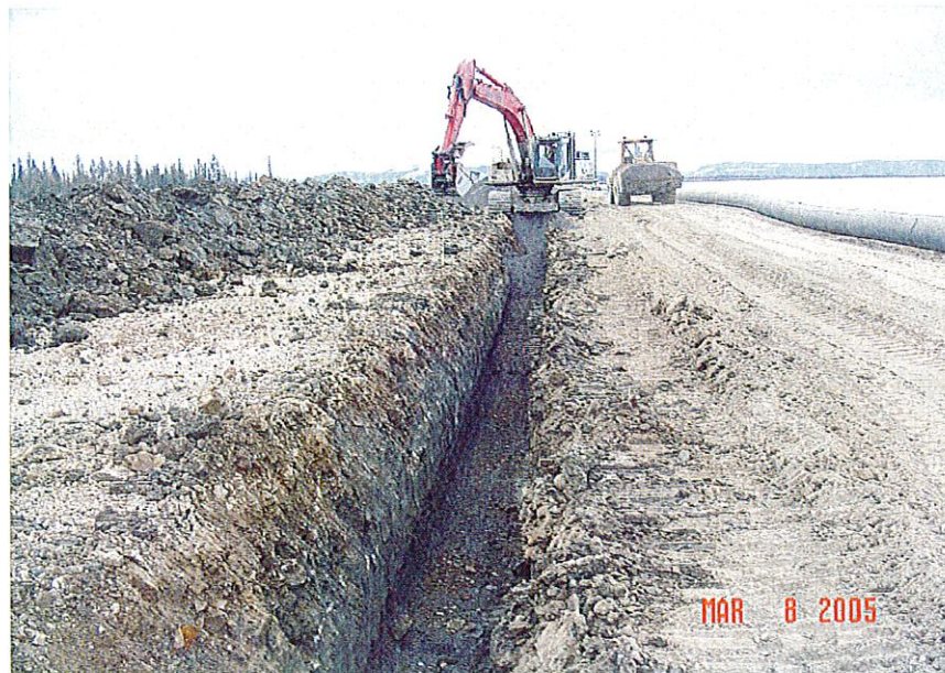
PHOTO 30 – Trench excavation for Zone F material and consequent filter placement with a loader.
