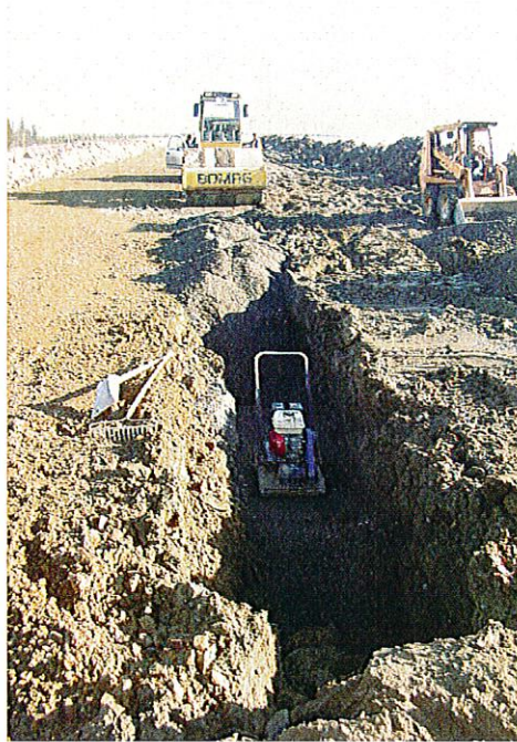
PHOTO 17 – Compaction of the Zone F material with hand-operated vibrating compactors a 10 tonnes vibrating compactor.
