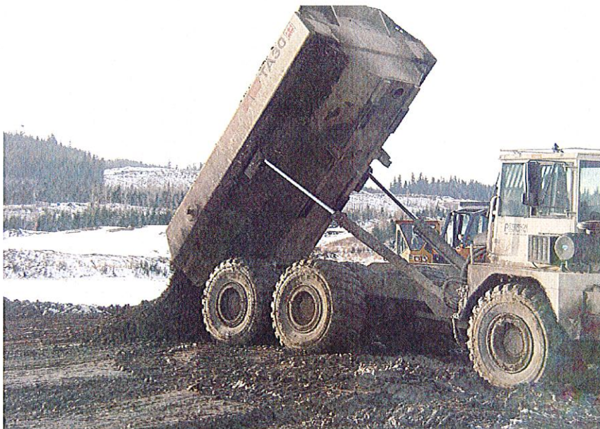
PHOTO 14 – Dumping Zone S material with a Terex dump truck with heated bucket during the cold weather.
