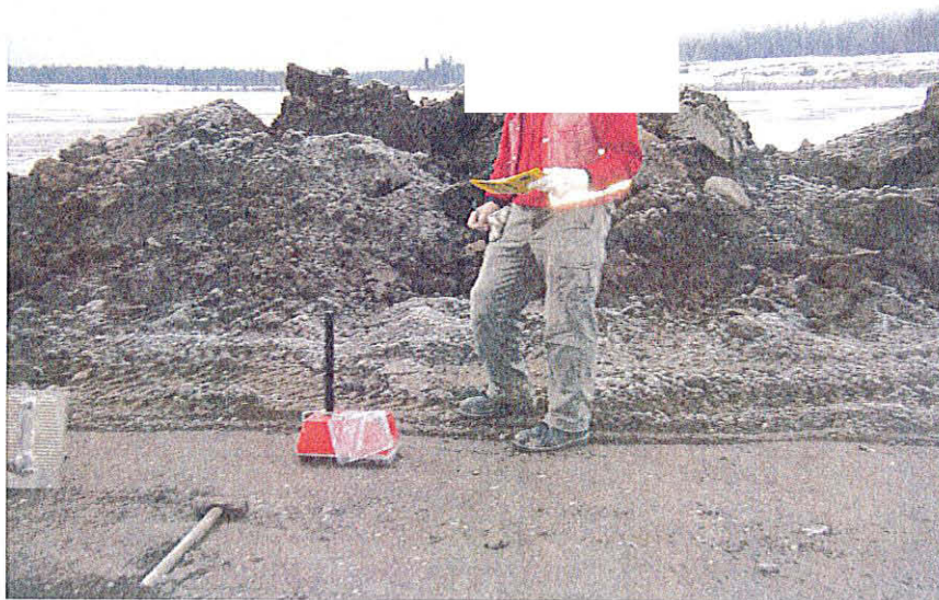
PHOTO 8 – Moisture and percent compaction control with nuclear gauge instrument by the Site Engineer.
