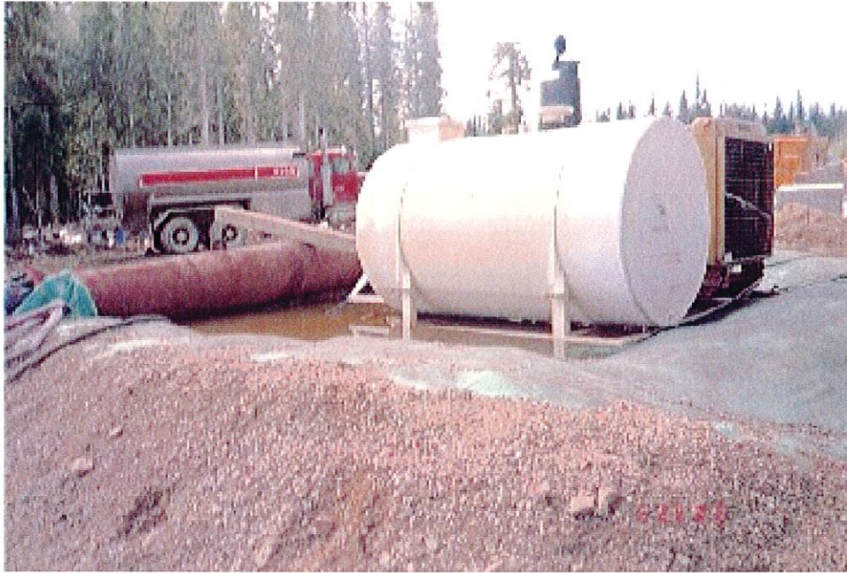
Photo No. 16: Polley Lake Pumping System.
