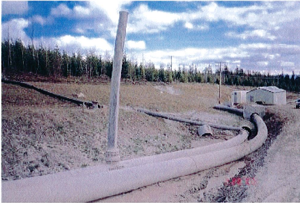
Photo No. 10: Tailings Pipeline with T2 Drop Box and Reclaim Booster Pump Station in background. Vertical pipe provides pressure relief, if required, during cycloning.
