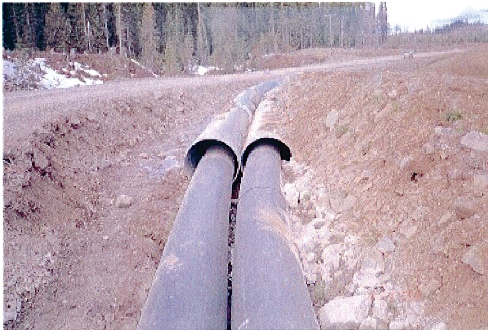
Photo No. 8: Pipeline Containment Channel. Downstream end of pipeline sleeves at Bootjack Creek Crossing.
