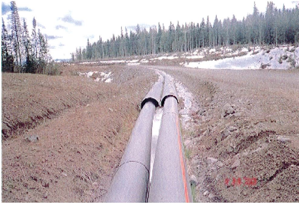
Photo No. 9: Pipeline Containment Channel. Upstream end of pipeline sleeves at Bootjack Creek Crossing. Minor amount of tailings at the bottoms of the sleeves.
