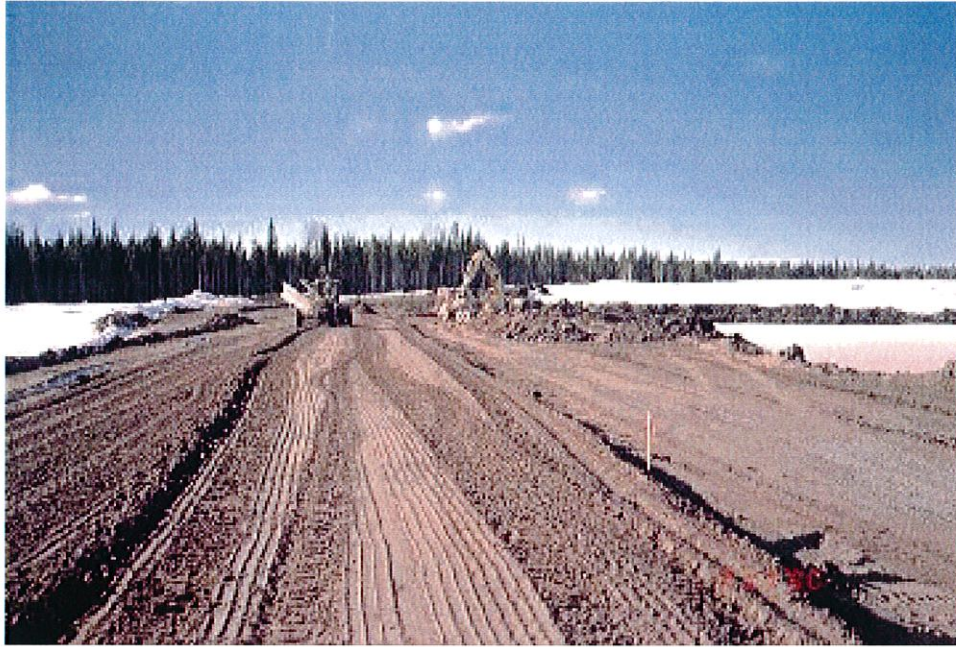
Photo No. 14: Mechanical placement of cycloned sand in the upstream fill of the Main Embankment.
