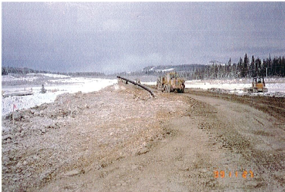
Photo No. 6: Perimeter Embankment upstream toe drain (to be installed later) will tie into the exposed pipe.
