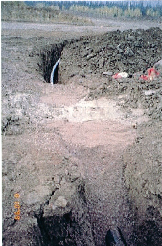
Photo No. 4: Upstream toe drain outlet. Backfill around the downstream seepage collars consisted of bentonite-modified till and filter sand.
