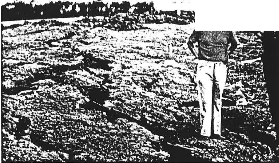
Damage behind the pitwall due to excessive blast charges per delay.
