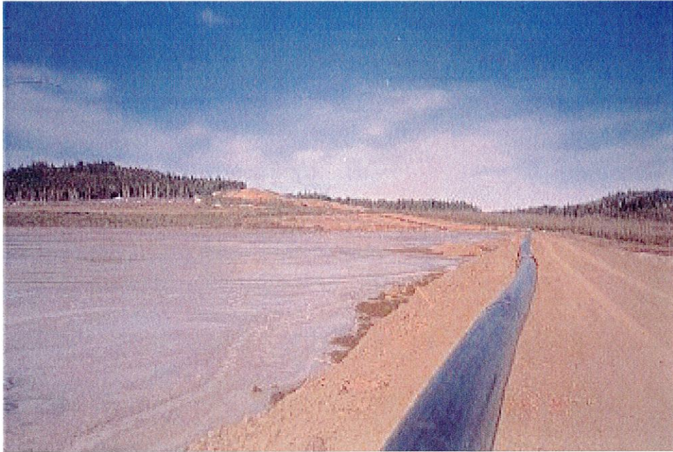
Photo No. 4: Perimeter Embankment, near CH 37+20 looking north. Note tailings beach development in northeast corner of the tailings impoundment.
