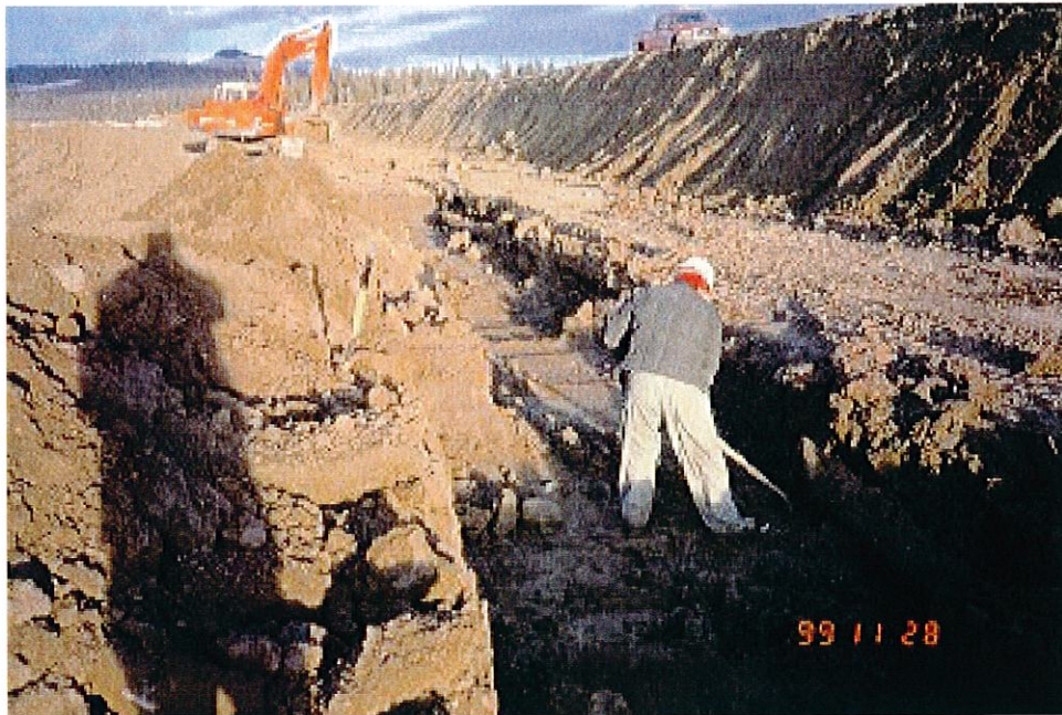
Photo No. 9: Trench for blank CPT pipe connecting Main and Perimeter Embankment upstream toe drains.
