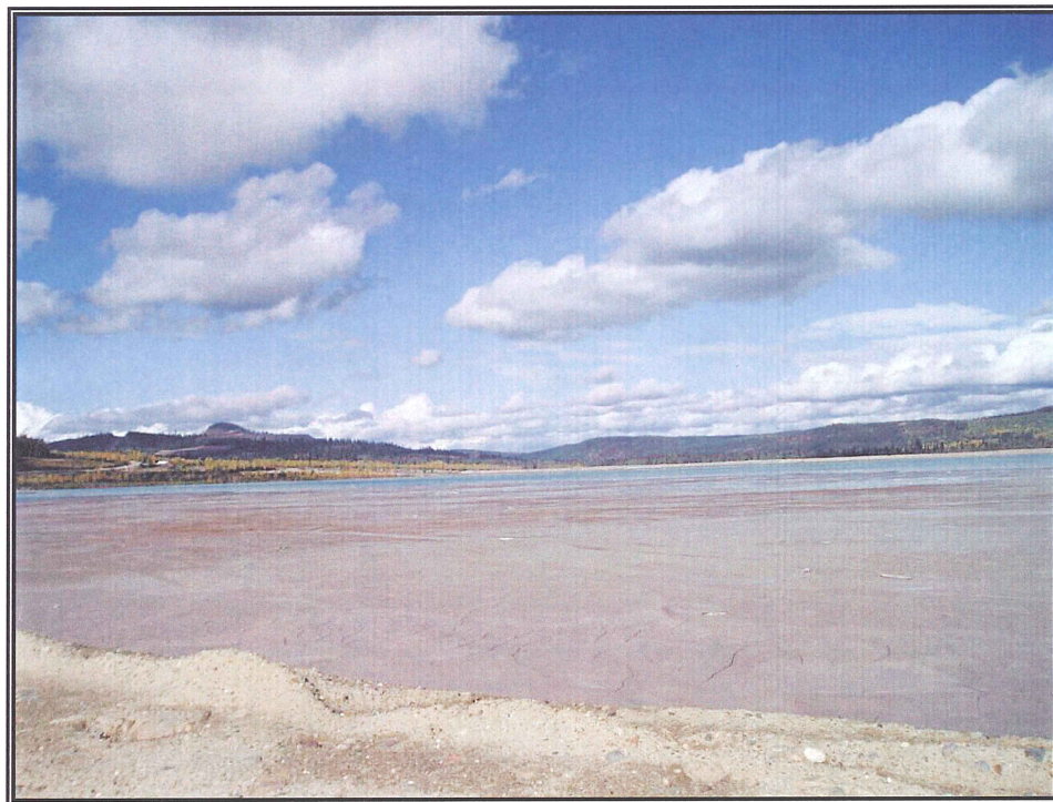
Photo 18: Minor Beach Development along Portion of Main Embankment
