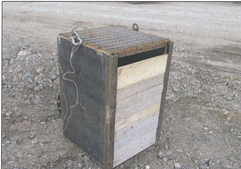
PHOTO 10 – Sand cell decant box.
