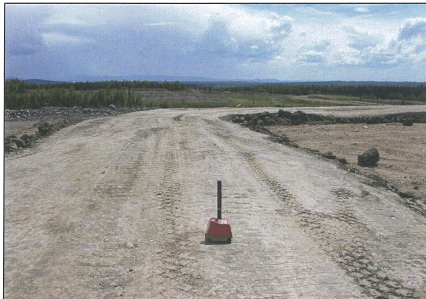
PHOTO 8 – Using the nuclear densometer to confirm field densities of Zone S material.
