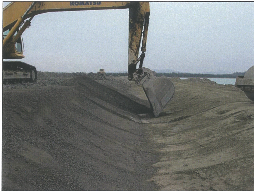
PHOTO 17 – Using a hoe to move the Zone F filter material into its final position.
