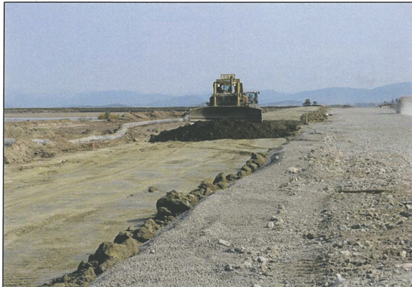
PHOTO 7 – Adding the 777's allowed for a second 'dozer roller team effectively doubling the till production rate
