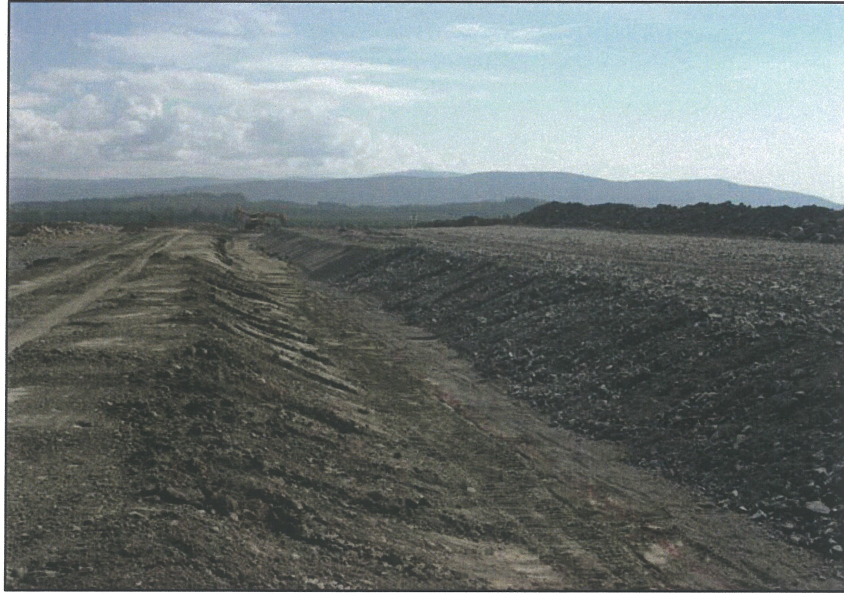
PHOTO 19 – Zone F Filter and Zone T transition material on the South Embankment.
