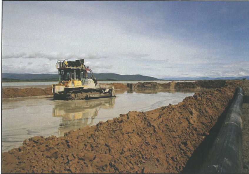
PHOTO 9 – Zone U sand Cell under construction decant box is shown in the background.
