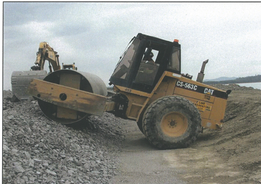
PHOTO 18 – Compacting the modified design Zone T. This new design is much faster and easier to compact.
