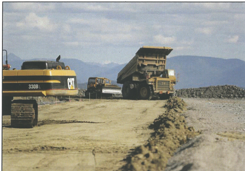
PHOTO 6 – Placing Zone S till material with mine fleet Caterpillar 777's near the end of the construction period
