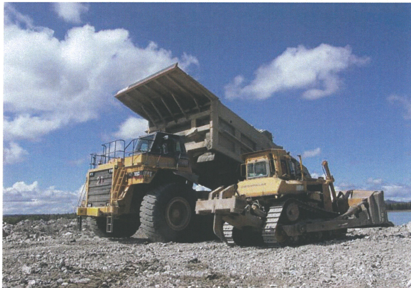
PHOTO 20 – Zone C consists of Non Acid Generating (NAG) waste rock from the pits brought to the dam by mine fleet trucks.
