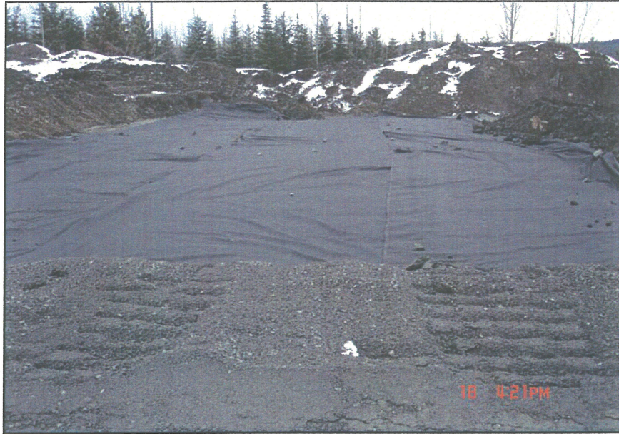
PHOTO 15 – Placement of geotextile cloth overtop of the original ground (competent till) prior to placement of Zone F material along the Perimeter Embankment
