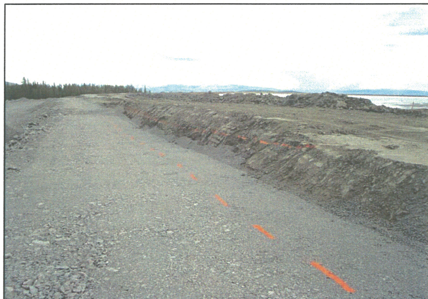
PHOTO 52 – Markings showing the ‘hoe’ operator exactly where to place the Zone F material against the Perimeter Embankment
