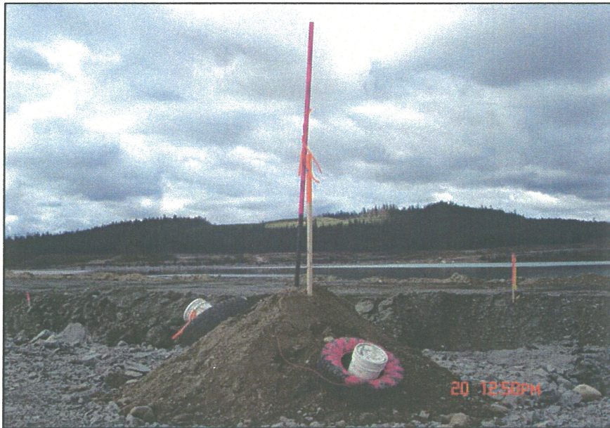
PHOTO 10 – Buckets and fluorescent poles act as protective measures to prevent damage to the new piezometers
