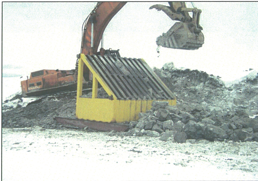
PHOTO 22 – Using the 'Grizzly' to filter the Zone T material, removing rocks greater than six inches in diameter
