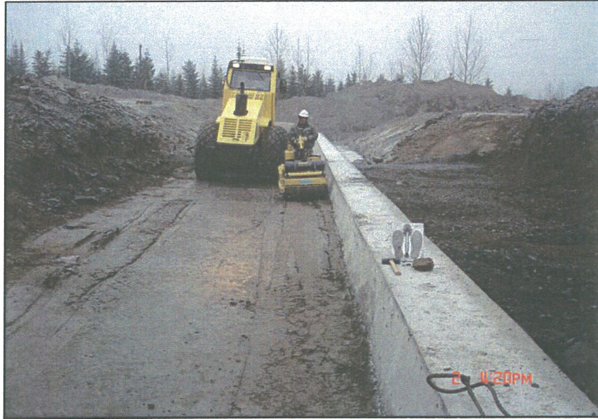
PHOTO 19 – Using the smaller packer to compact the Zone S right up against the encasement, and the 10-tonne vibrating drum roller for the remaining area
