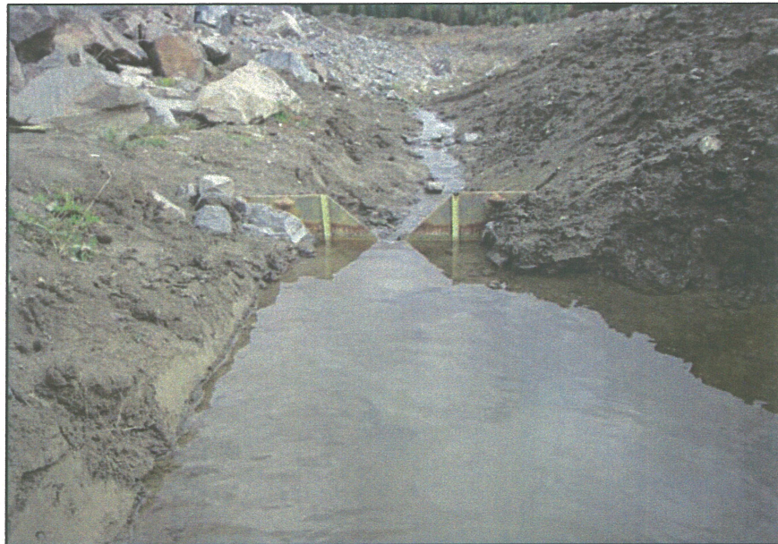
PHOTO 34 – Tape measures installed at the Main-South Embankment corner weir to provide an efficient means of determining the height above the V-notch.
