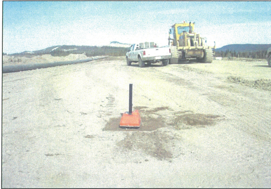
PHOTO 53- Performing a compaction test on the Main Embankment U zone with the nuclear densimeter.
