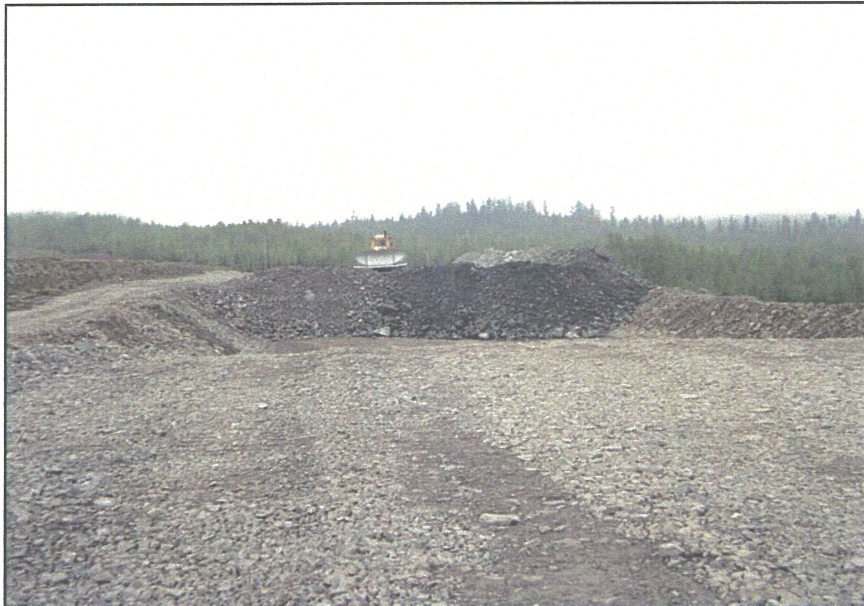
PHOTO 50 – Placement of Zone C in three meter lifts along the Perimeter Embankment.
