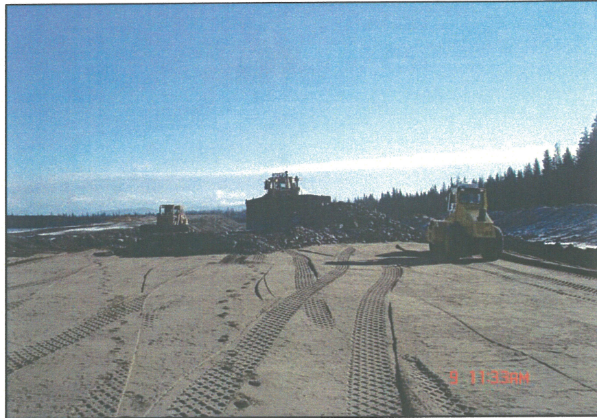
PHOTO 39 – Placing Zone T material overtop the Zone FT material, prior to placement of Zone C along the South Embankment.
