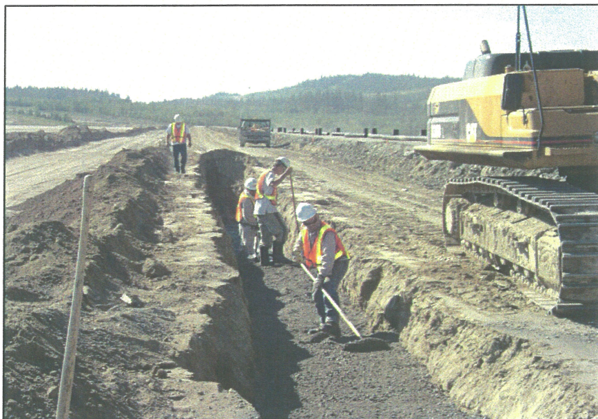
PHOTO 13 – Contractors leveling the Zone F material prior to placement of the Perimeter Embankment Upstream Toe Drain
