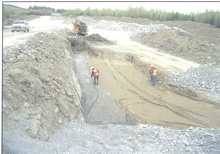
PHOTO 51 – Excavating to ‘competent till’ north end of the Perimeter Embankment. The area downstream of the Zone F region was excavated to original ground, and Zone FT was placed overtop, after which Zone T was placed.
