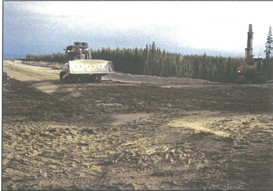
PHOTO 47 – Placement of Zone S material on the South Embankment, the last section to be brought up to elevation 951 m with Zone S.
