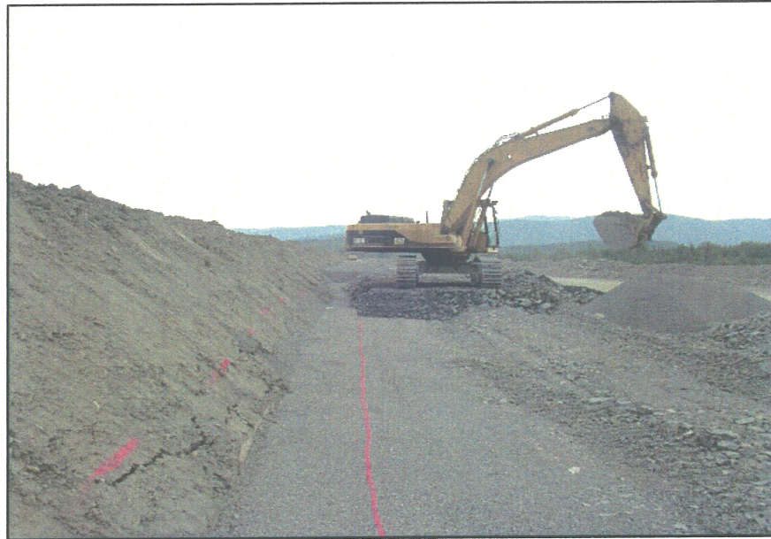
PHOTO 45 – Placing Zone T material along the South Embankment, leaving a one meter section for the Zone F.
