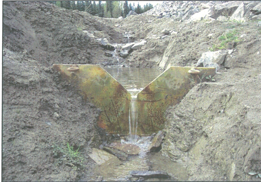
PHOTO 33 – V- notch weir used to measure flows at the corner downstream of the Main and South Embankments.
