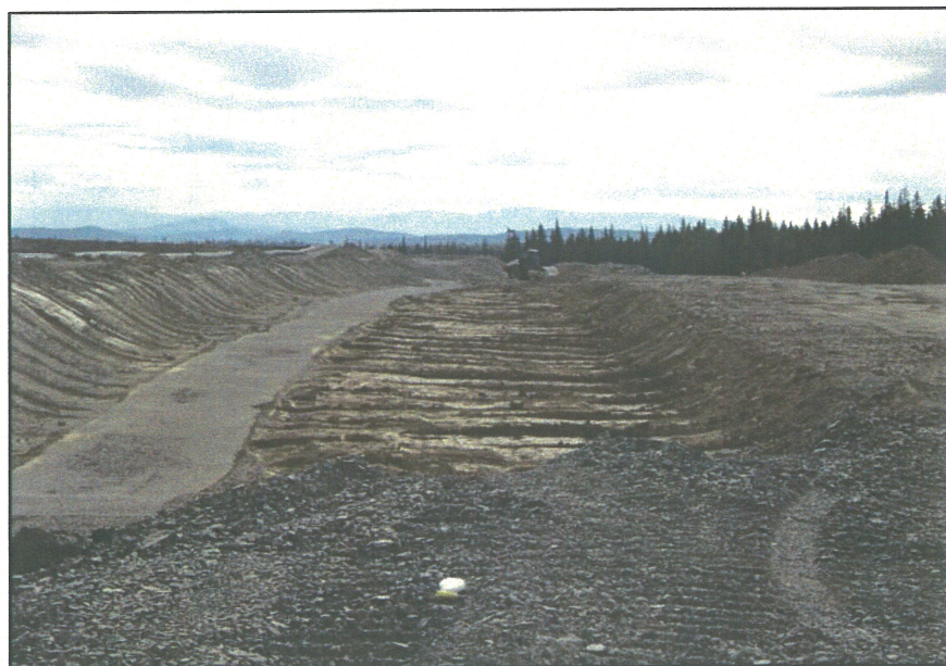
PHOTO 42 – The foundation drain in place and backfilled with Zone F material. The area downstream of it was excavated to original ground, and covered with Zones FT, T, and C.
