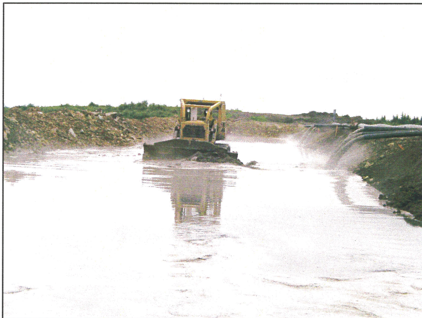
PHOTO 10 – Using a dozer in the sand cell at the South Embankment to distribute and compact the tailings sand.
