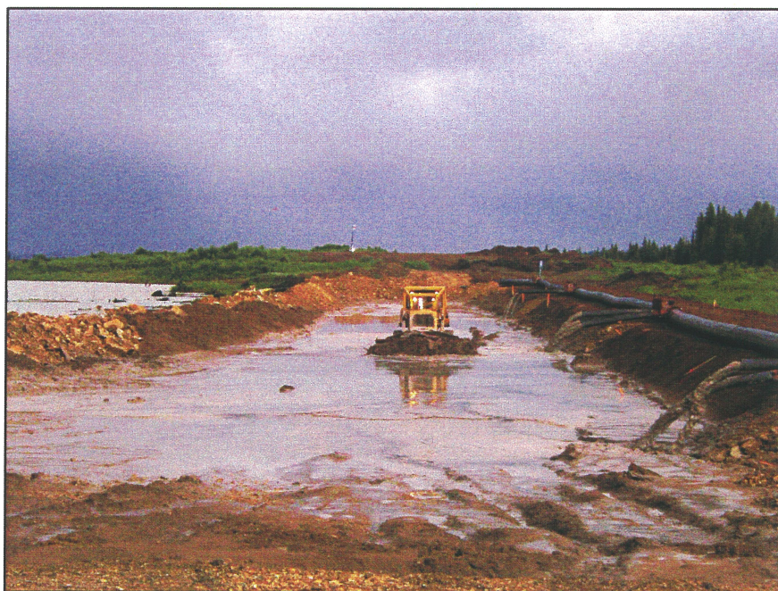
PHOTO 11 – Using a dozer in the sand cell at the South Embankment to distribute and compact the tailings sand.
