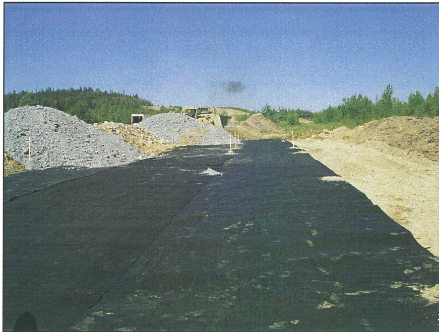
PHOTO 4 – Geotextile placed on the Perimeter Embankment prior to placement of the shell zone.
