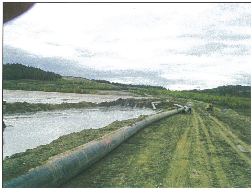
PHOTO 16 – Sand cell on the Perimeter Embankment. Tailings are discharged at the far end and exit into the TSF through culverts installed at the opposite end of the cell.
