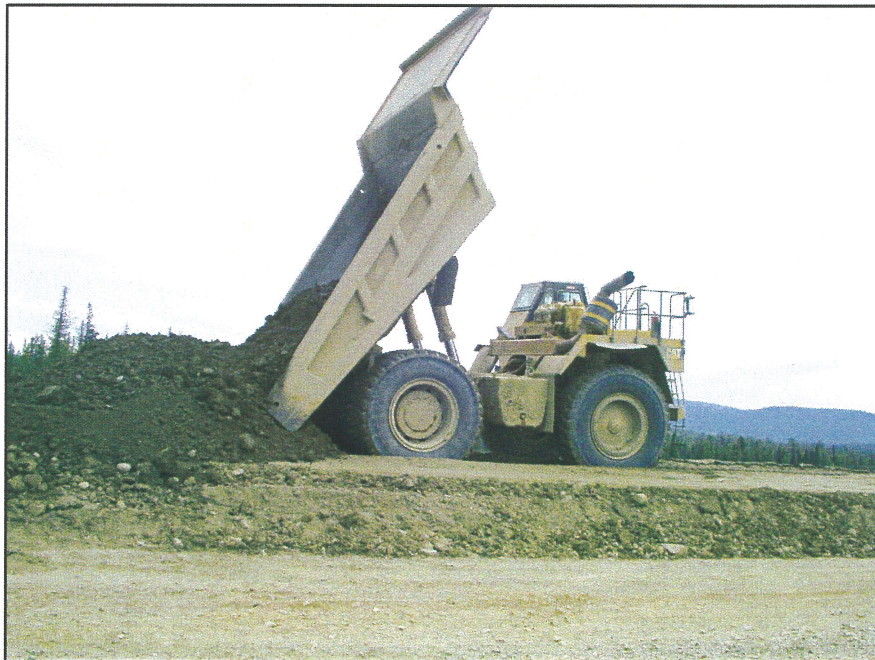
PHOTO 28 – Placing Zone S material with a 777 haul truck on the Perimeter Embankment.
