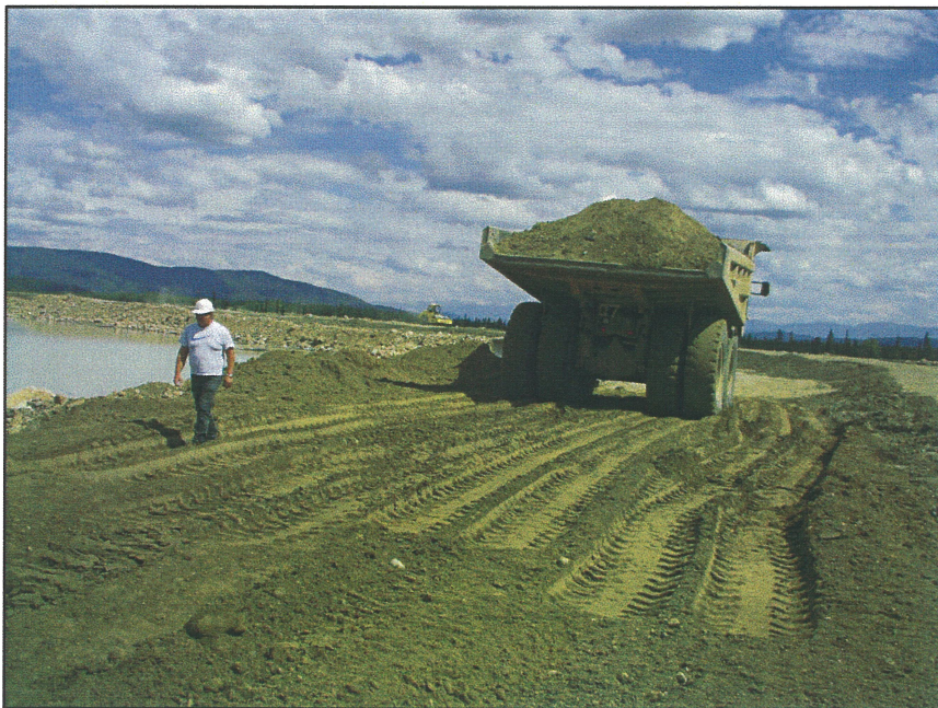
PHOTO 30 – Placement of Zone U material on the Main Embankment. The Zone U material for the Main Embankment was sourced from Borrow Area No. 3.
