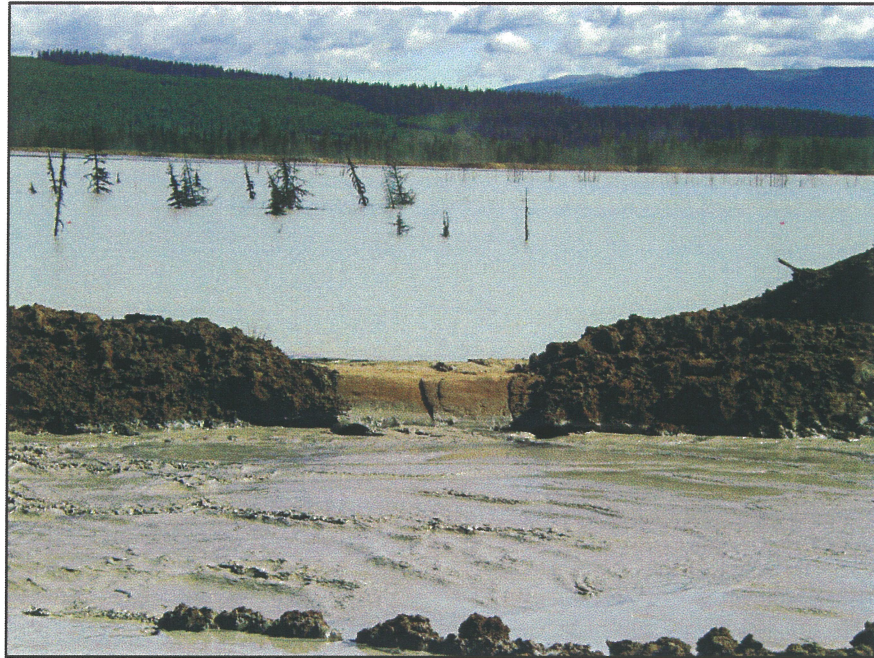
PHOTO 13 – Typical sand cell drains, which are raised as the sand elevation rises.
