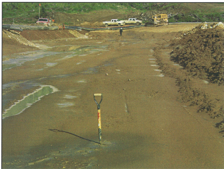
PHOTO 12 – 0.3 m of sand was placed in 7.5 hours in the first sand cell at the South Embankment.
