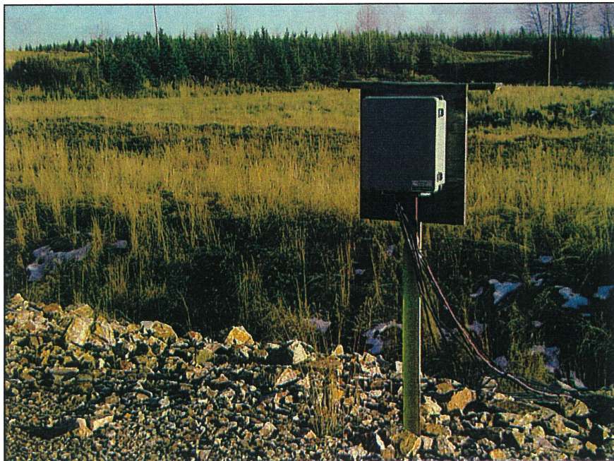
PHOTO # 14 – SINCO Terminal Panel for Piezometers
