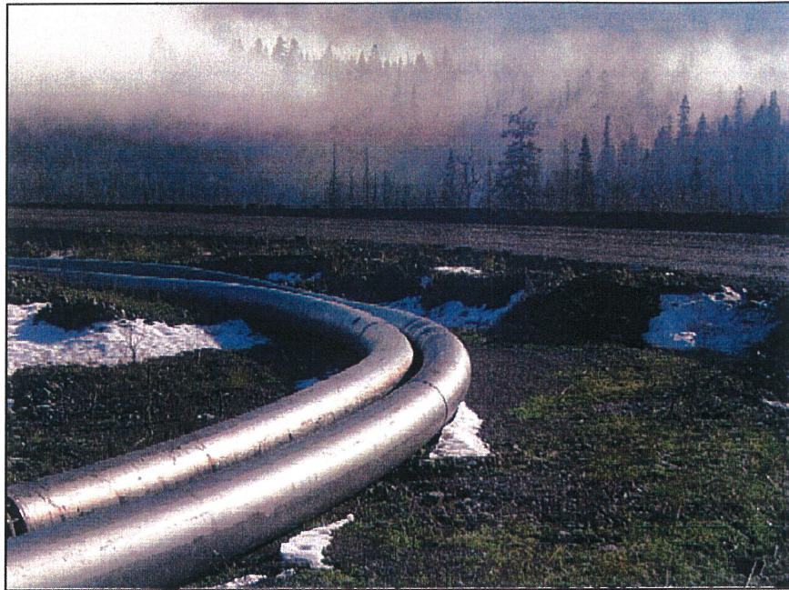
PHOTO # 3 – Tailings and Reclaimed Water Pipelines (View 1)
