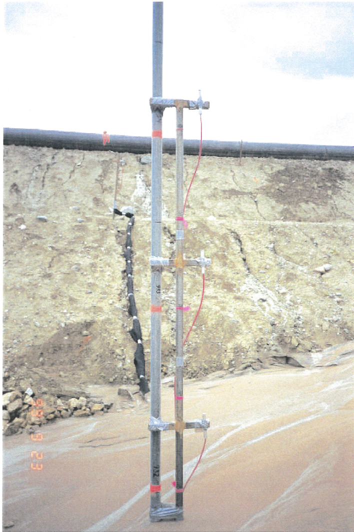
Photo No. 3: Downstream Trial vibrating wire piezometer post.
