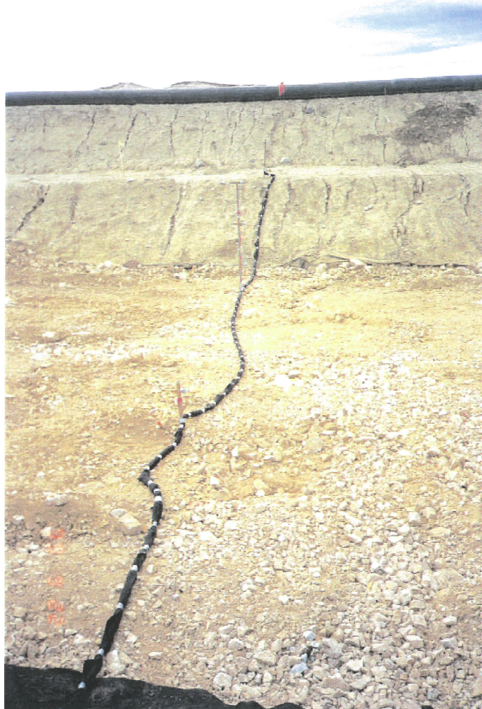
Photo No. 2: Downstream Trial vibrating wire piezometers. Leads wrapped in geotextile fabric for protection.
