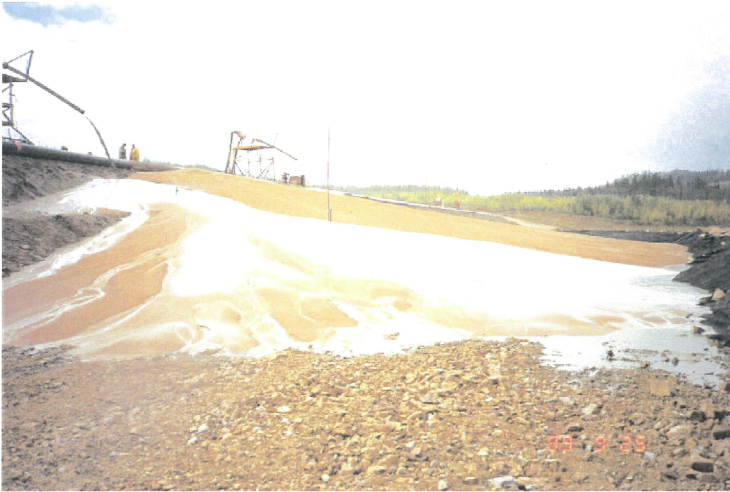
Photo No. 4: Downstream Trial – Phase I cycloned sand deposition. Note upstream face of rock berm covered with geotextile fabric.
