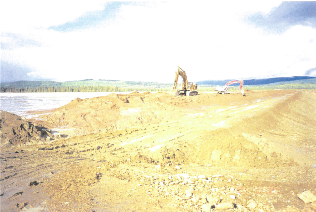
Photo No. 2: Main Embankment Upstream Trial Berm - Excavation for upstream toe drain.
