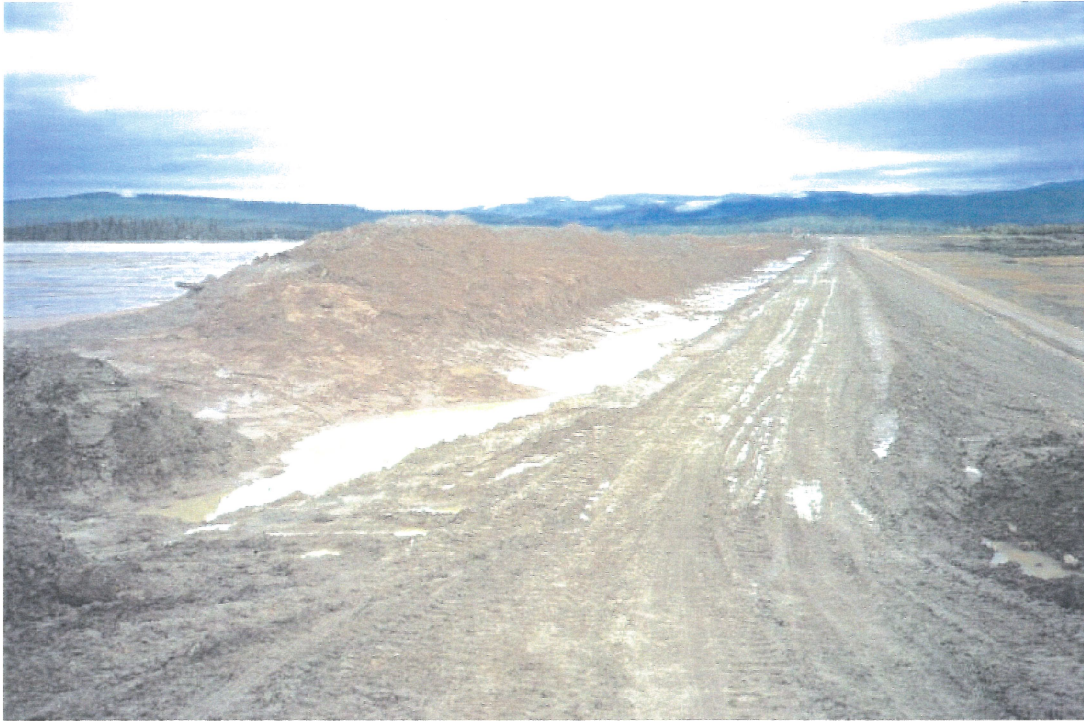
Photo No. 3: Main Embankment Upstream Trial Berm and upstream toe drain ditch.
