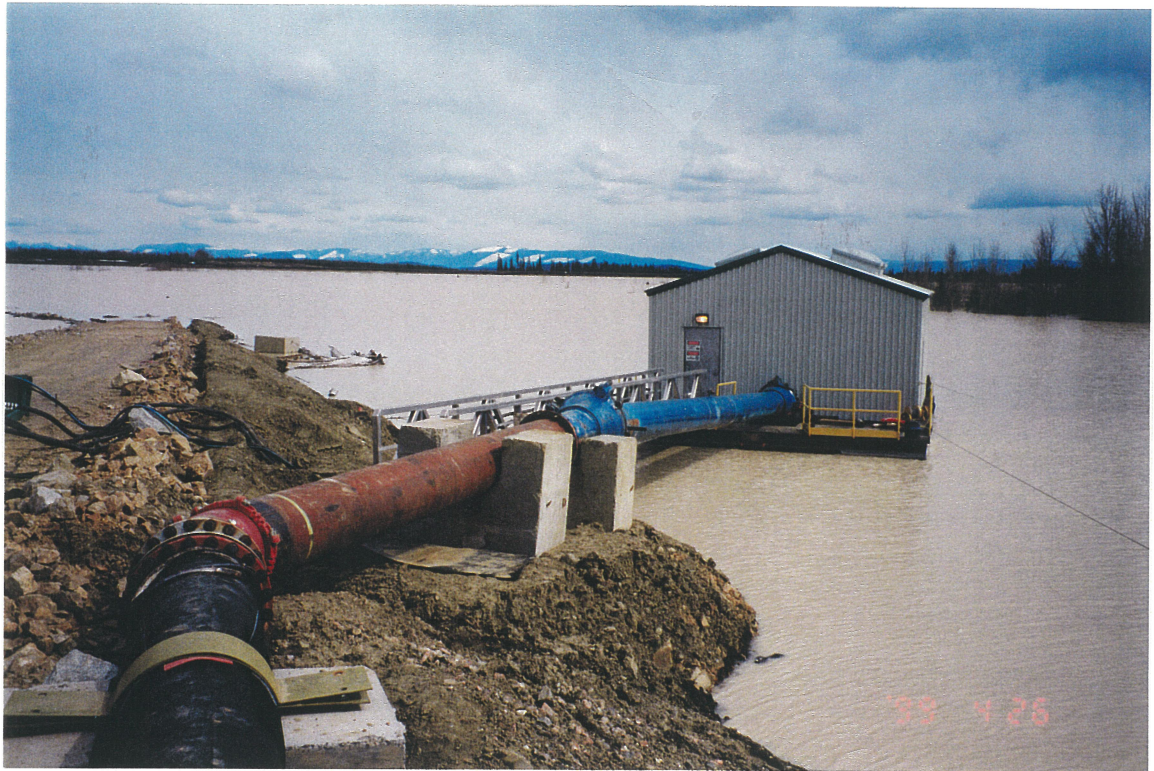
Photo No. 14: Reclaim Pipeline System. Reclaim Barge and Channel. Note 35 degree elbow added and barge alignment changed.
