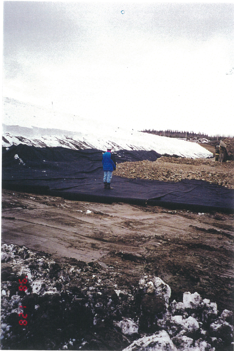
Photo No. 3: Prepared foundation at Perimeter Embankment with Type 2 Geotextile Filter Fabric layer between Transition Zone Material (Zone T) and Foundation Soil, January 28, 1998.
