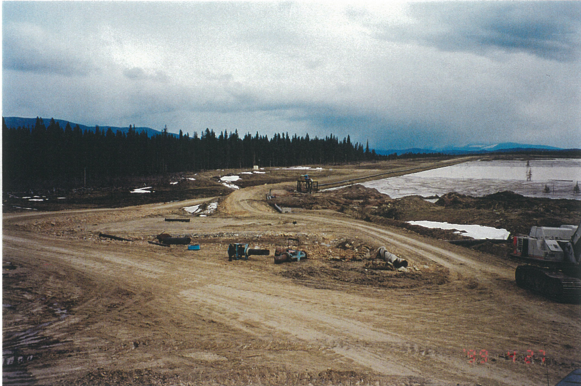
Photo No. 4: Perimeter Embankment from left abutment. Note tailings beach development and set-up of 60 inch cyclone.
