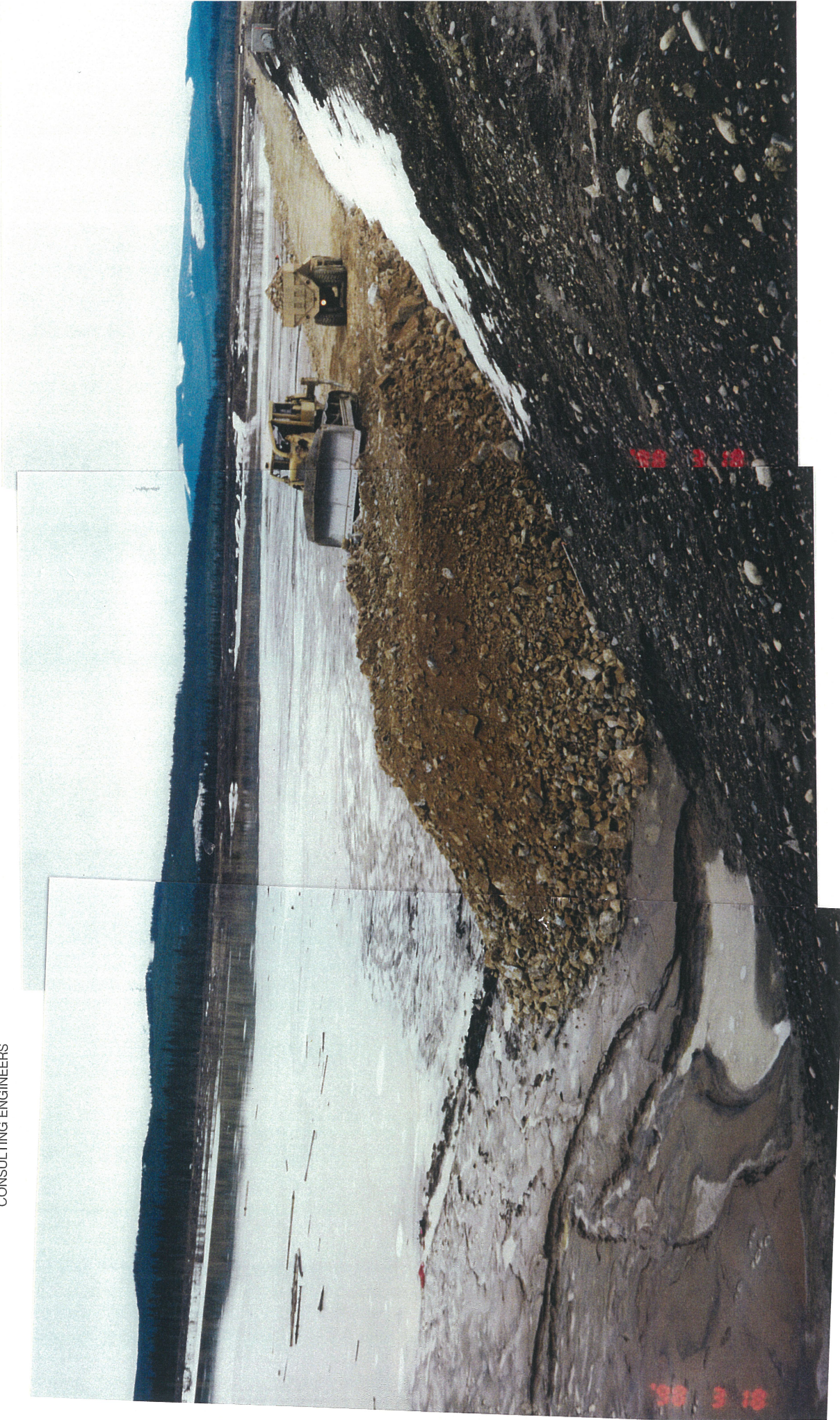
Photo No. 5: Placement of Coarse Bearing Layer (Zone CBL) on Tailings at Main Embankment, March 18, 1998.
