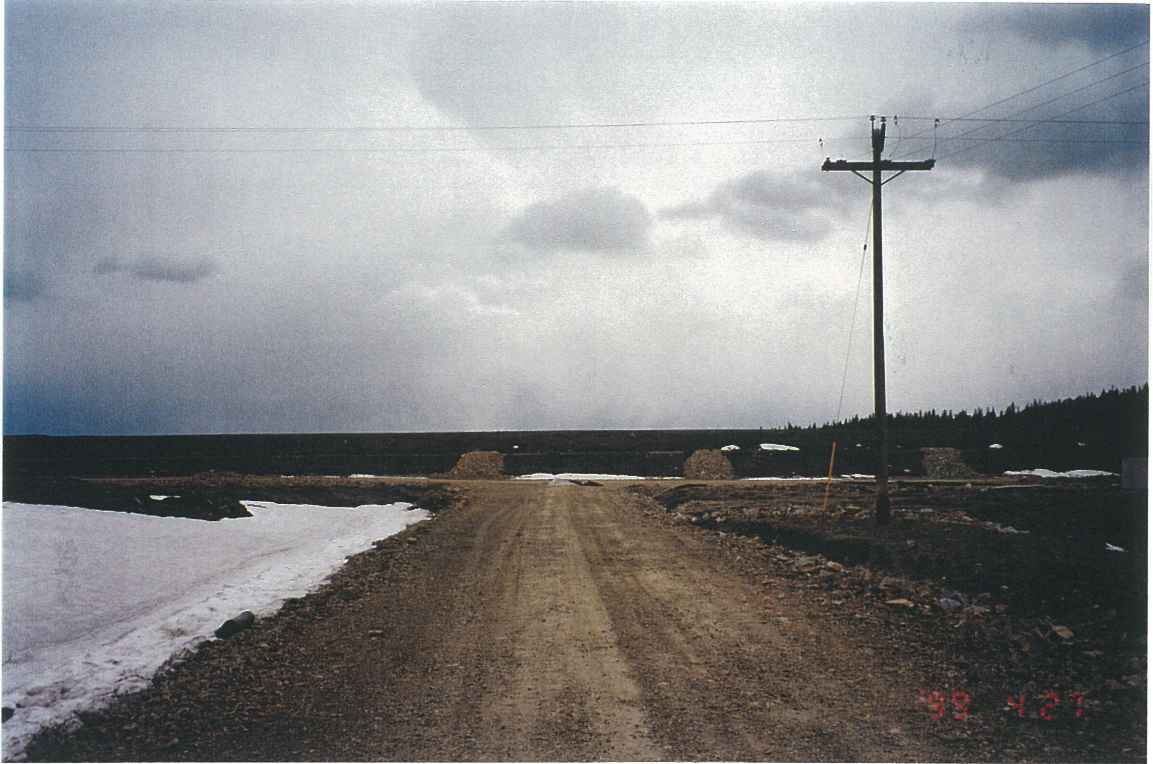
Photo No. 6: Perimeter Embankment. Looking upstream from access road on east side of Seepage Collection Pond. Note Outlet Drains going up face of embankment.
