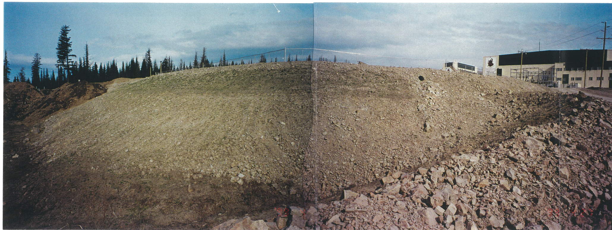
Photo No. 21: Millsite Sump. View of south slope, looking west. Slope is stable. No seepage observed.
