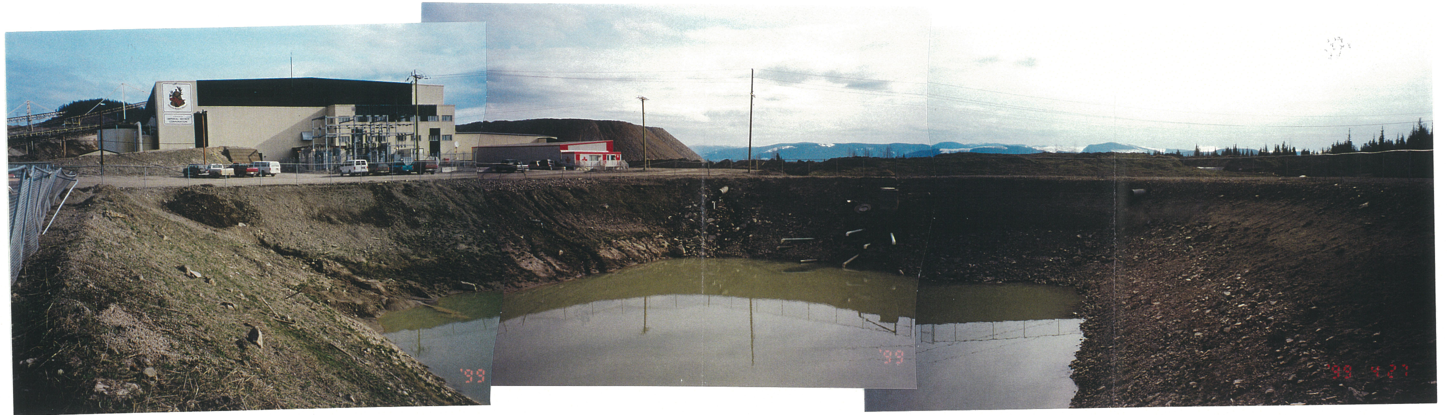
Photo No. 20: Millsite Sump. Note low water level and stable inner slopes.
