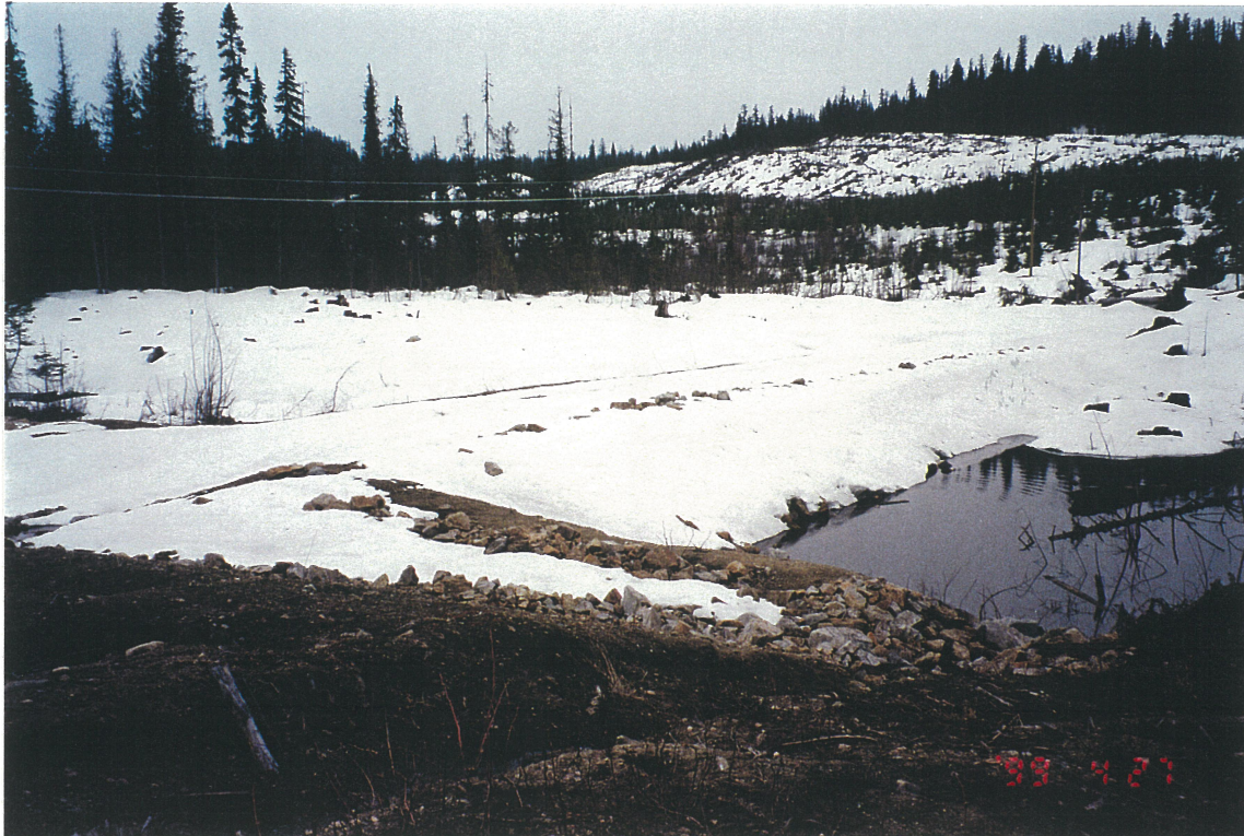
Photo No. 22: South Bootjack Dam. View of upstream face of embankment, looking northwest. Ponded water is now seeping through old dam back into Bootjack Lake.
