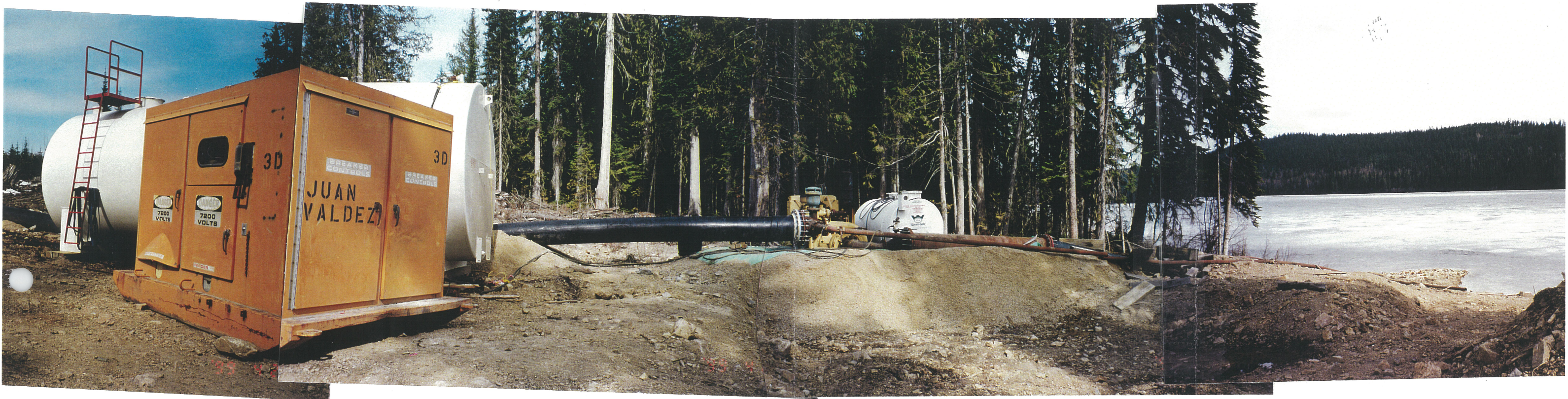
Photo No. 19: Polley Lake Pumping System. Intake Area. Note float on Polley Lake. Float is attached to the intake.
