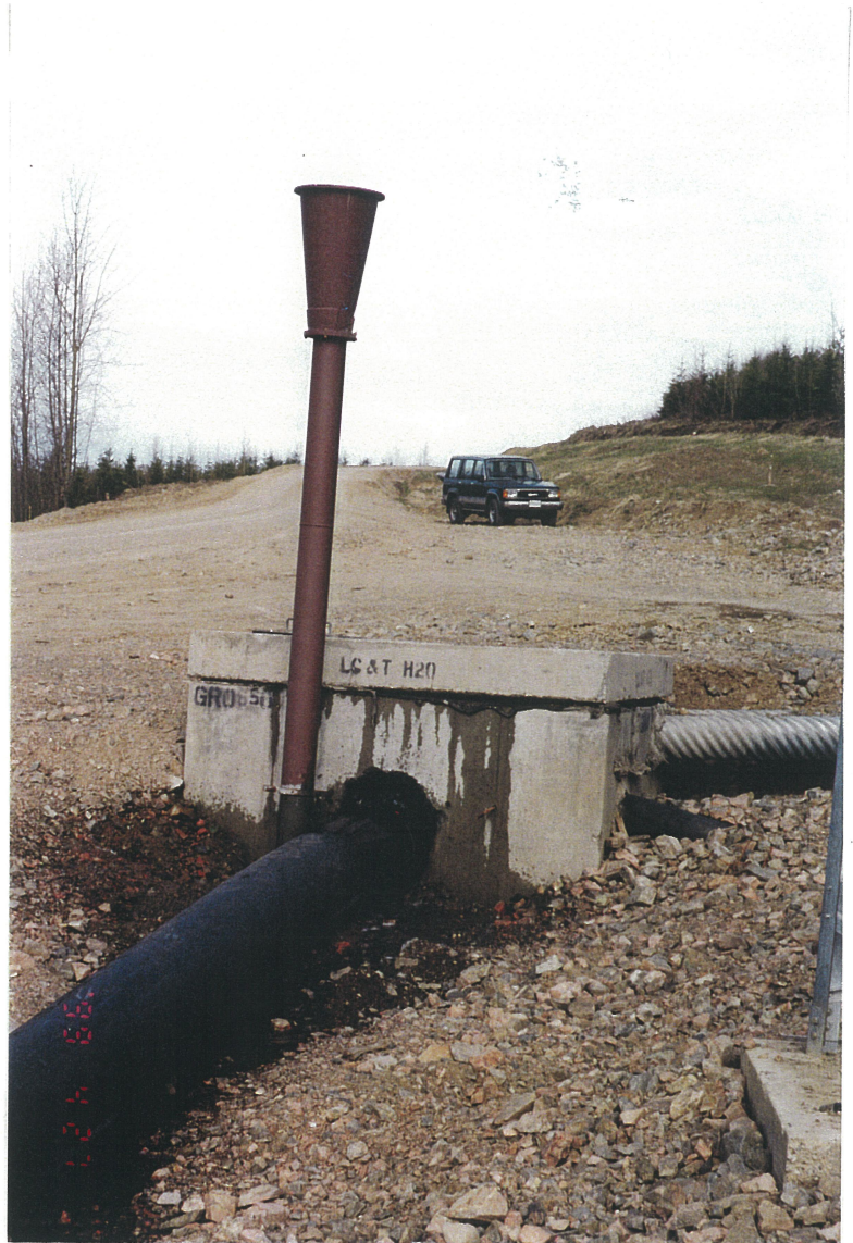
Photo No. 12: Tailings Pipeline System. Revised T2 Dropbox. Tailings Pipeline now extends all the way from the Mill to the Tailings Storage Facility. T2 Dropbox provides surge protection and is connected to the pipeline by a bifurcation.
