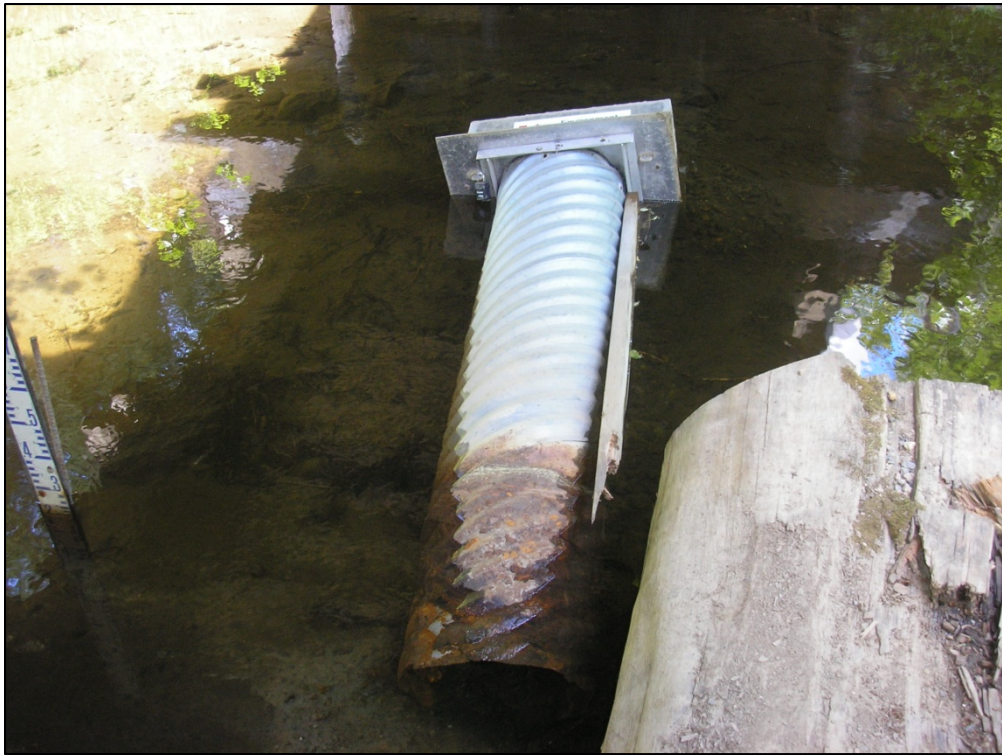
Photo 3: Water Survey of Canada chart recorded hut after pushed into Hazeltine Creek. Photo taken July 6, 2010.
