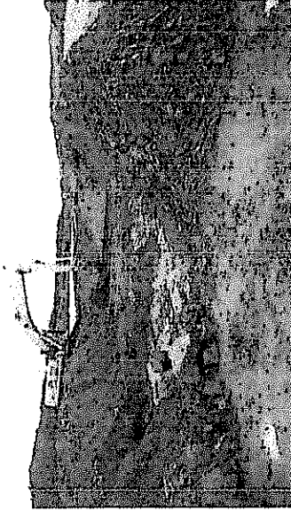
Photo 8: Establishing a temporary berm at perimeter pipe crossing due to weather on May 28
