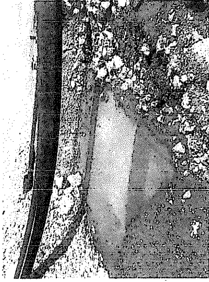
Photo 3: Standing water over the core at perimeter pipe crossing on May 27th
