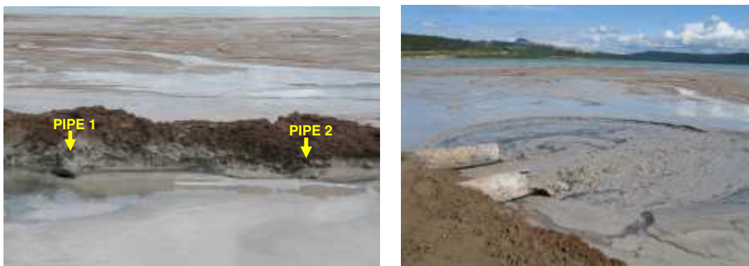
Photo 5 – Cell decant system
