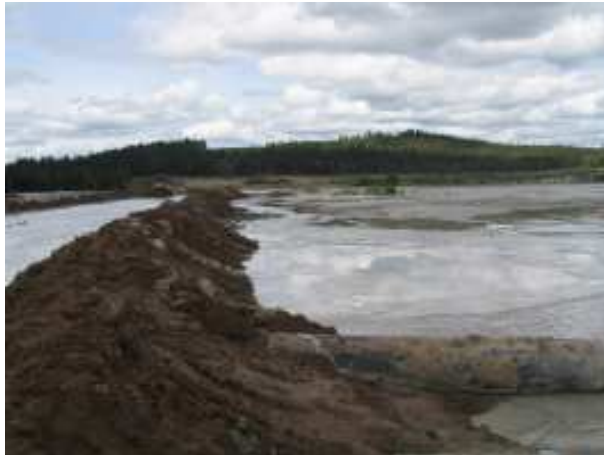
Photo 6 – Berm erosion by decant channel flow
